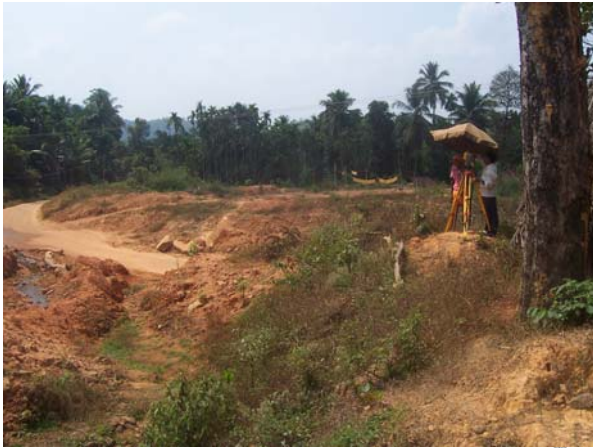
Photo 15: Heaped up material at toe may act as natural barrier for future.
