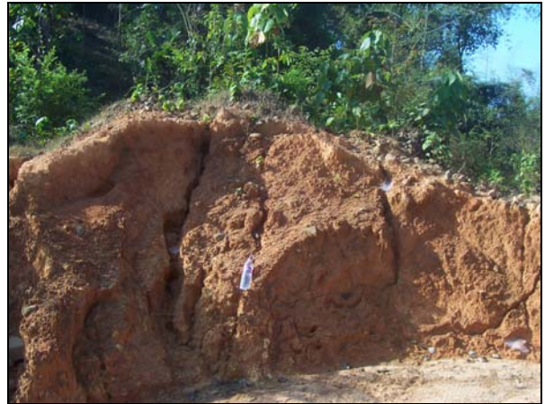
Photo 14: Gully erosion in the zone of depletion.
